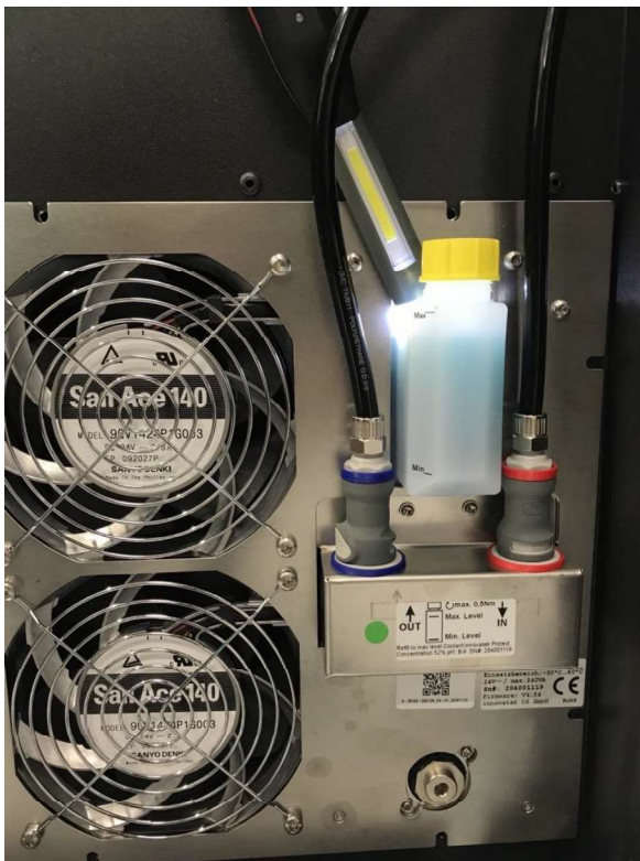
Figure 83: Checking the cooling liquid level
