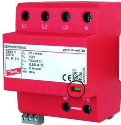
Figure 80: Check of overvoltage protection
