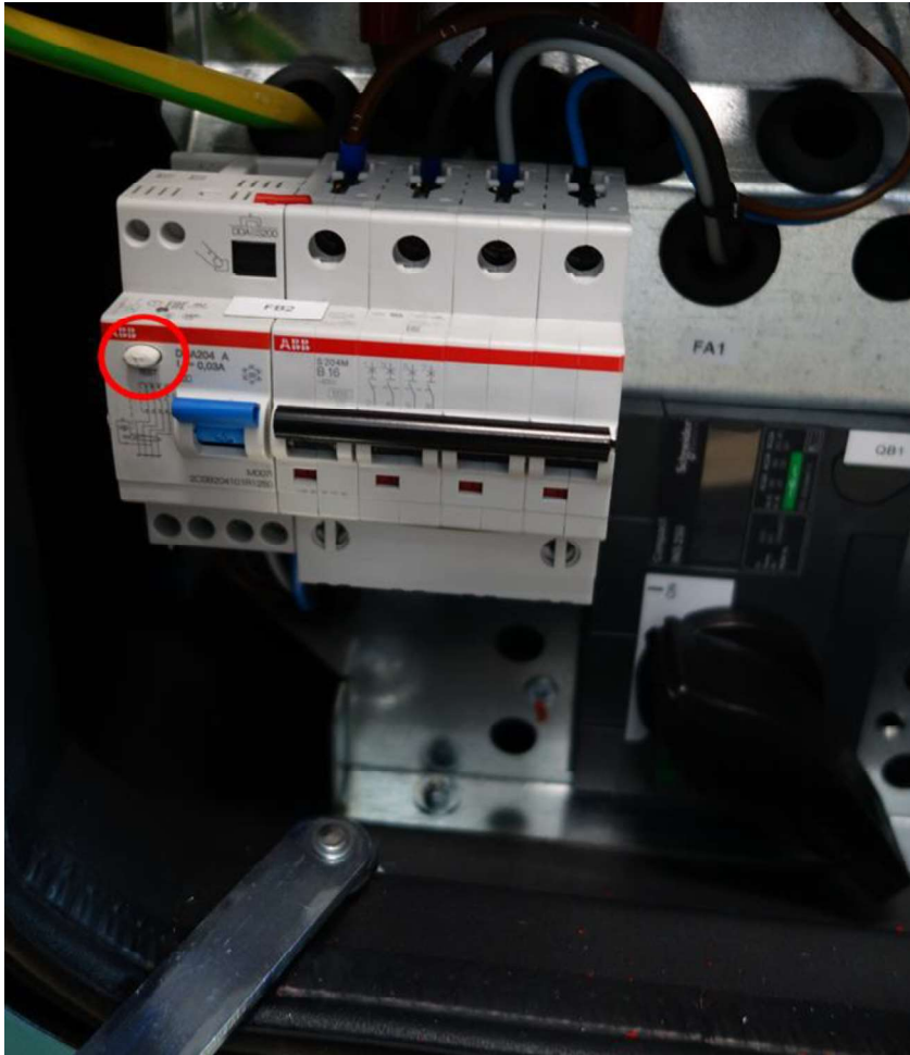
Figure 77: Function test of the circuit breaker
