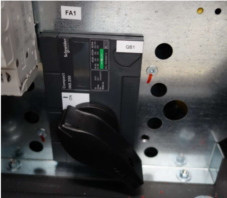
Figure 78: Function test of main switch
